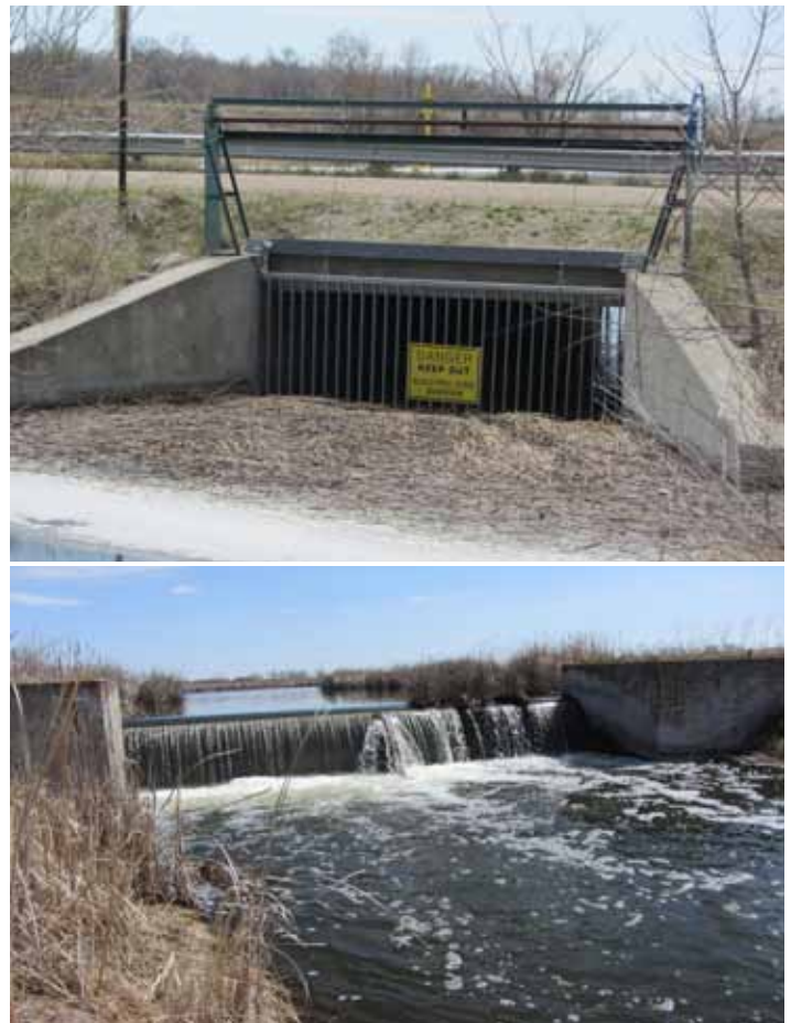
Figure 14. (top) The electric barrier on Lake Christina. The screen is dammed up with lake debris in the spring. (bottom) A carp dam downstream of Pelican Lake on Pelican Creek. Credit DNR SHP.
